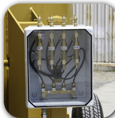
Safety Operator Control Valves
